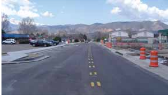
York Road, looking west, shows the new curb and gutter, sidewalks, and future entrance to the new Earl Drive and Woodmen Valley Shopping Center.
