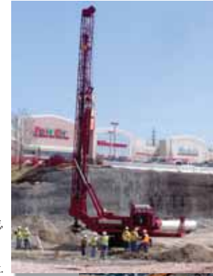
LEFT: Bridge construction begins with the drilling of caisson holes for the foundation support. The drill pictured (or another like it) will be used to drill a total of 54 caissons. The hole diameters range from 30 inches at the abutments to 36 inches under the columns. Rebar "cages" will be placed inside the 35-foot-deep caissons and then backfilled with concrete.
